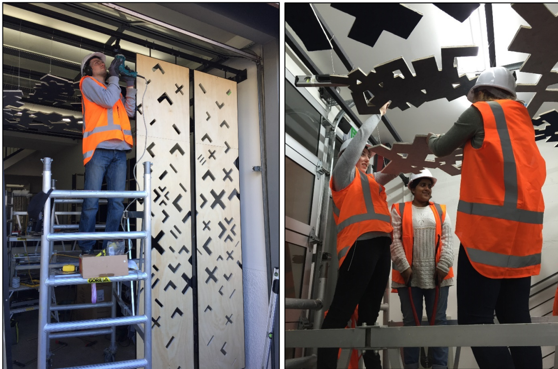
Figures 7a: Installation of privacy screens (left). Figure 7b: Installation of the acoustic cloud panels (right). Photos: Contractor, Janus and Patel (2016).
